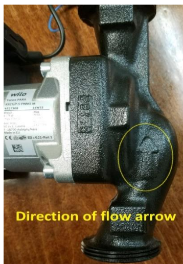
Verify flow direction (UP)
