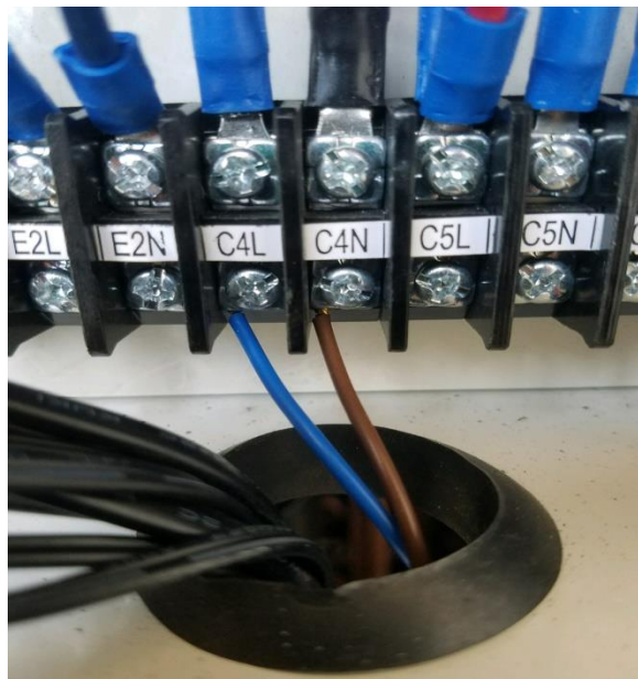
Pump power wires.
